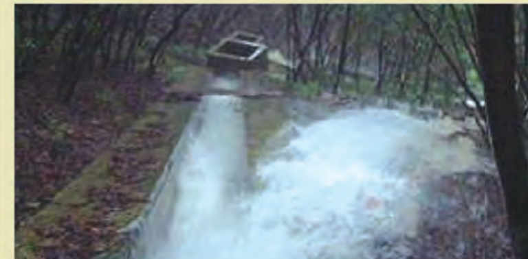
Figure 2 Spillage or overflow of drainage channels
