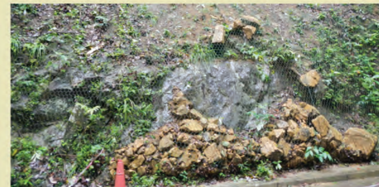
Figure 4 Rock debris retained by rock mesh
