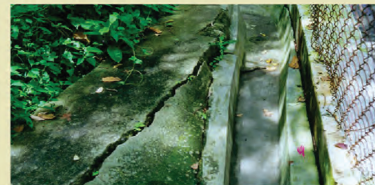
Figure 3 Widening of cracks
